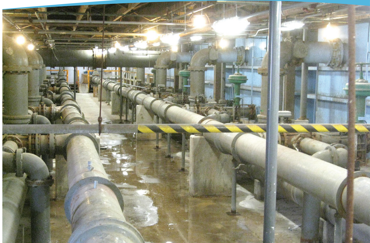
▲ New lighting system at the water plant is first step in overhauling some of the plant's electrical service.
